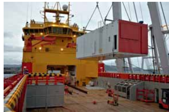
The 320 kW “HotModule” fuel cell from MTU Onsite Energy was installed on board the Norwegian offshore supply ship VIKING LADY in September 2009.
